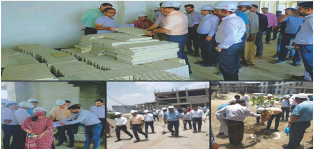
Mr. Rajesh Kumar Yadav, Joint Secretary, DEPwD and Dr. Honnareddy N., Director NIMHR visit at NIMHR construction site
