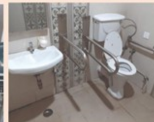
Accessible Toilet with grab-bars
