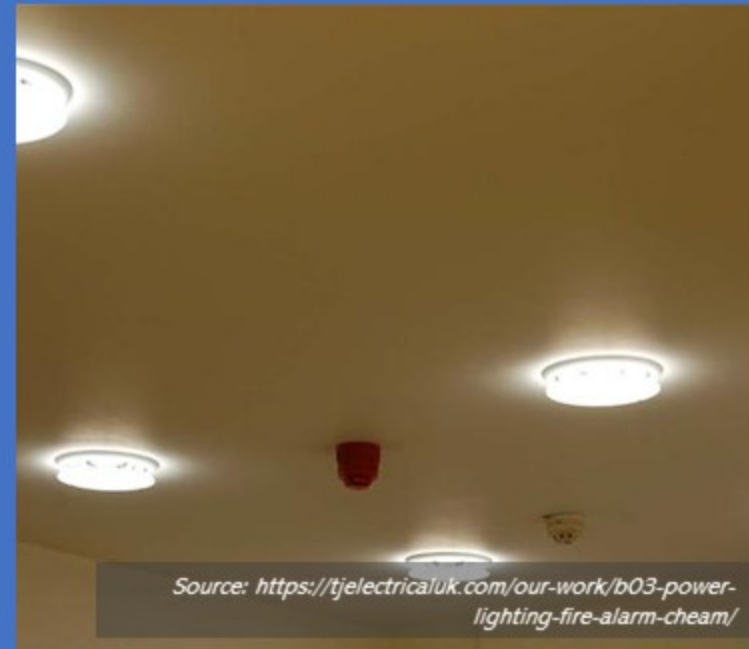
Flashing Beacon as a fire alarm system
