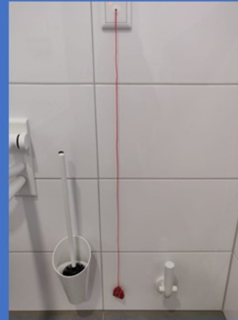
String type alarm system
