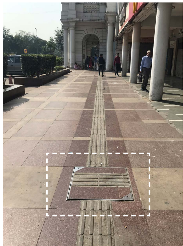
Image 2.20 Inconsistent laying of tactile guiding tiles
