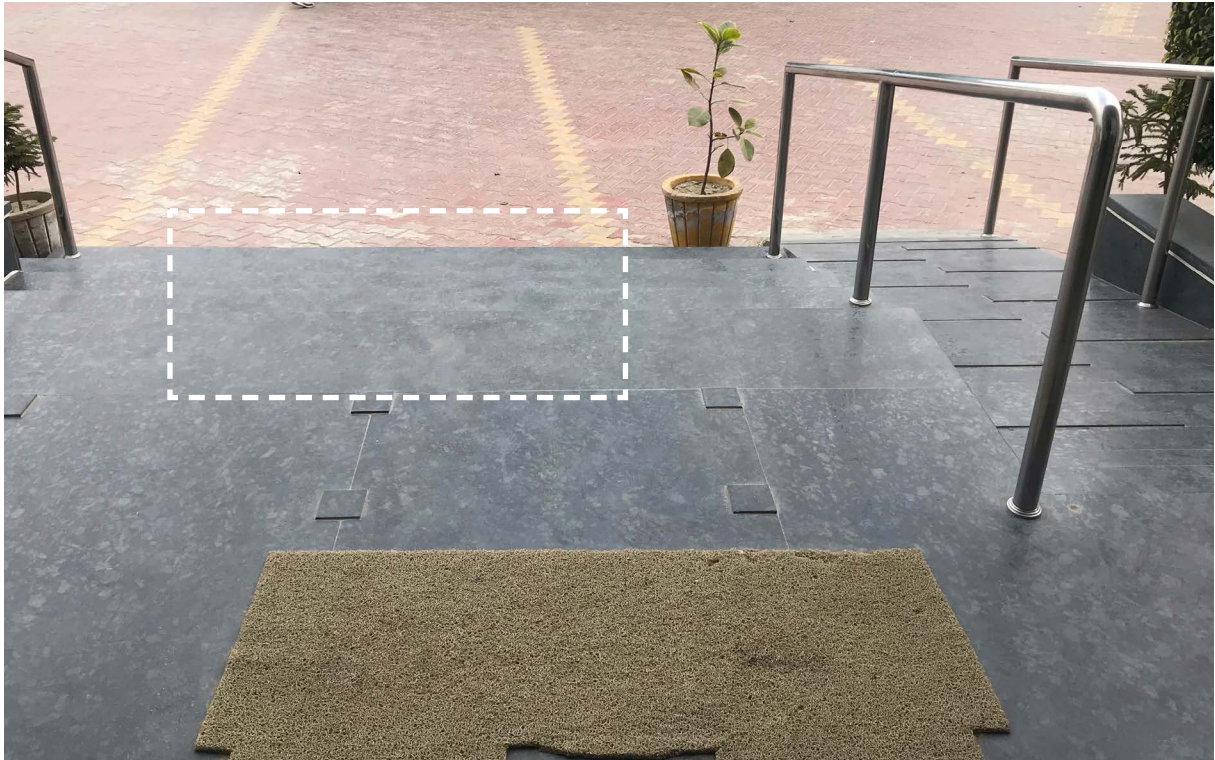
Image 2.18 Poor visual contrast in entrance steps
