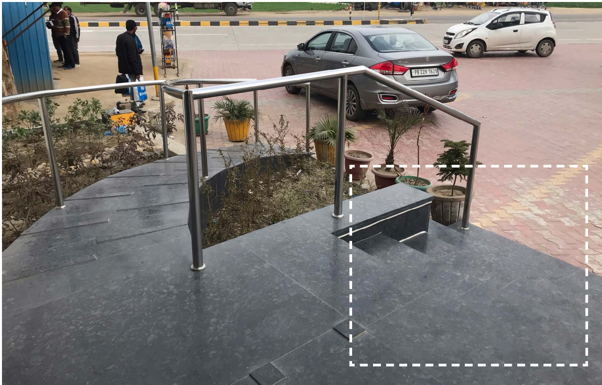
Image 2.10 Inadequate visual contrast
