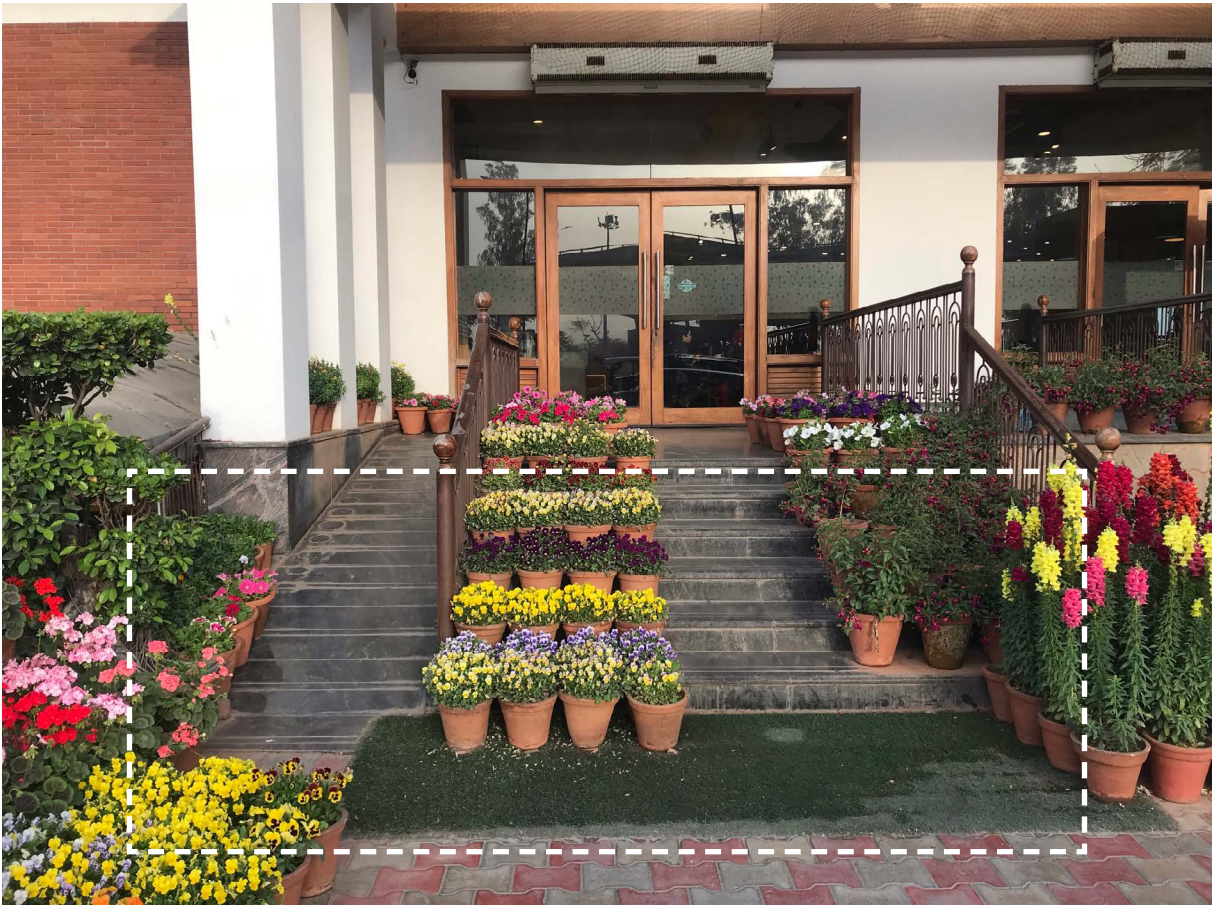
Image 2.12 Planters as barrier and inadequate ramp slope
