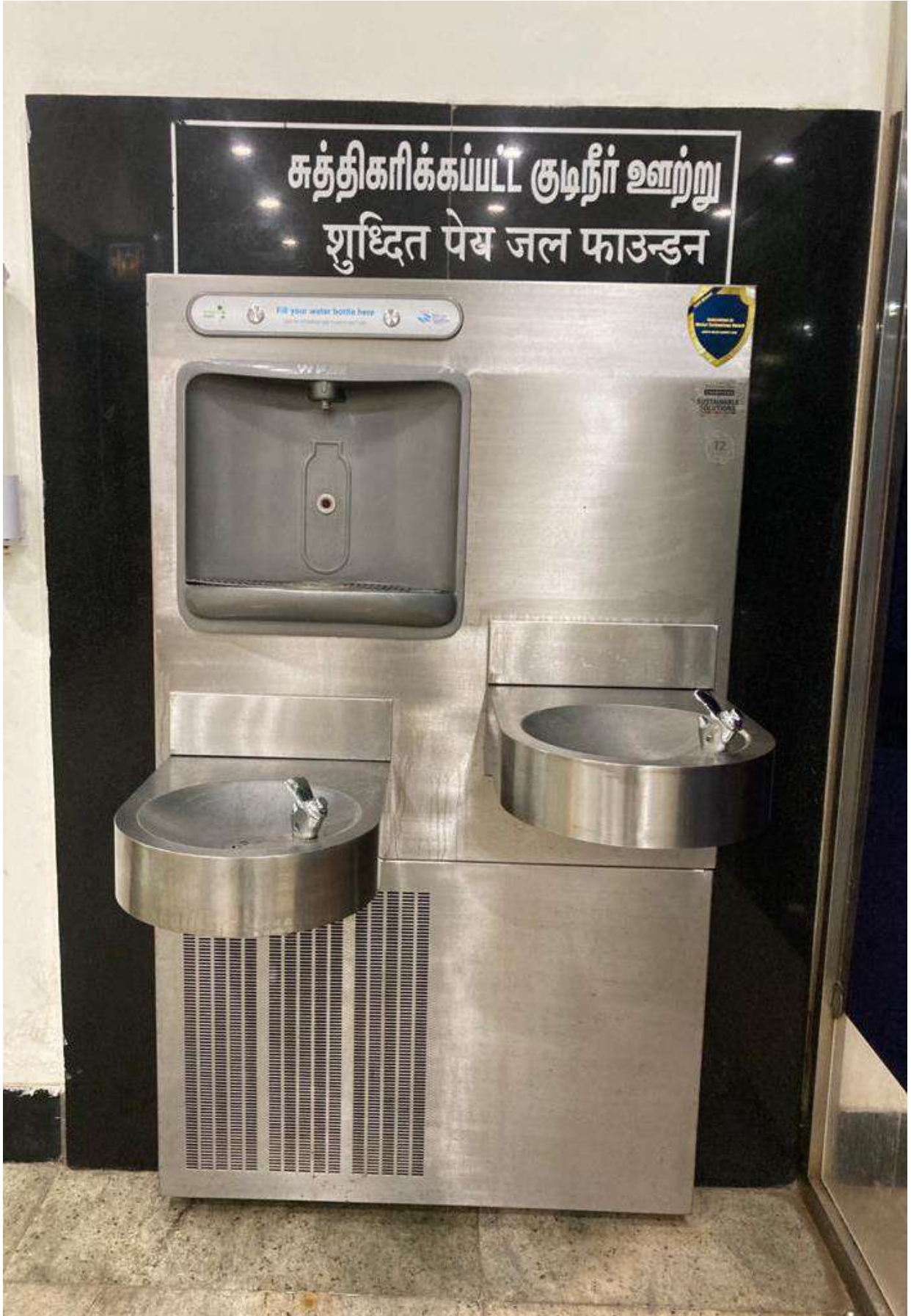
Image 16: Example of Drinking water facility with taps on two levels installed in Madurai Airport
