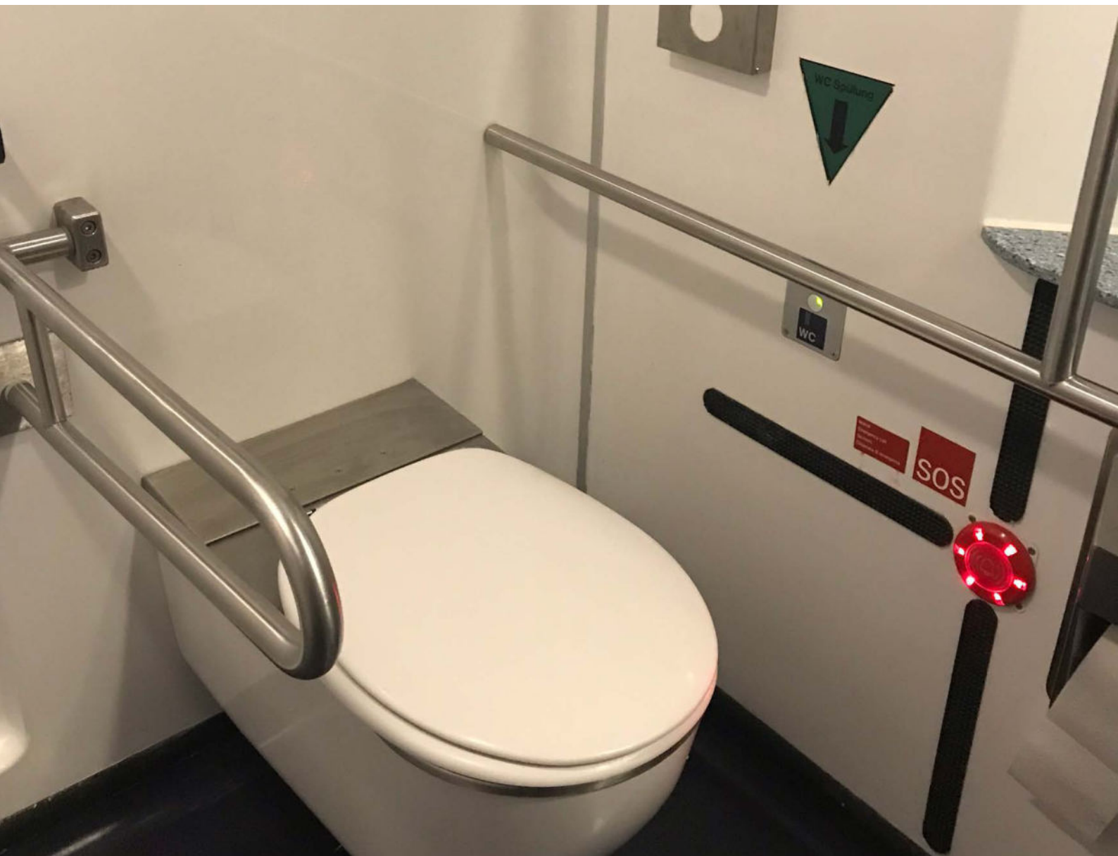
Image 4.25 Accessible Washroom with SOS facility Photo Credits: Dr. Gaurav Raheja
