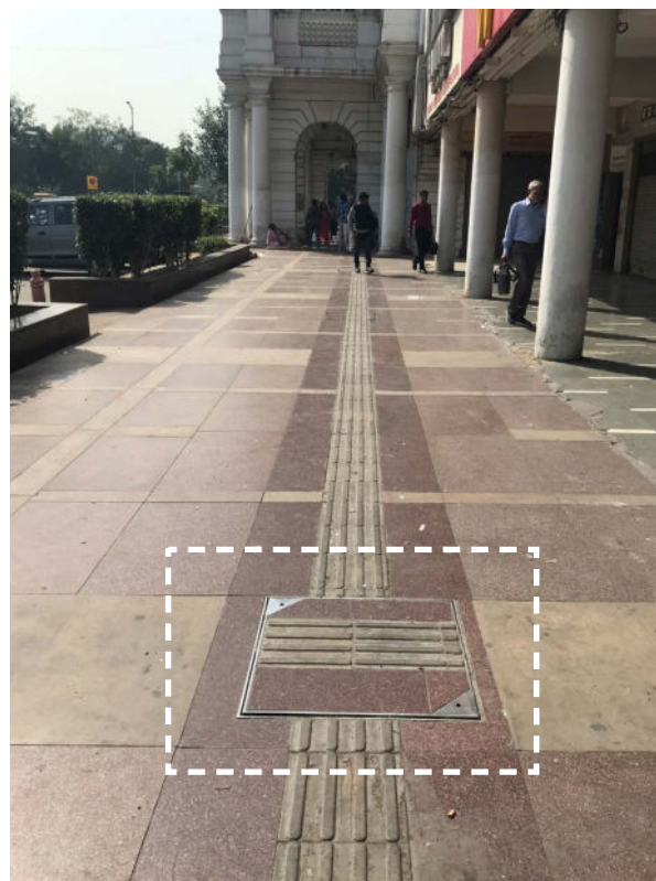
Image 2.20 Inconsistent laying of tactile guiding tiles
