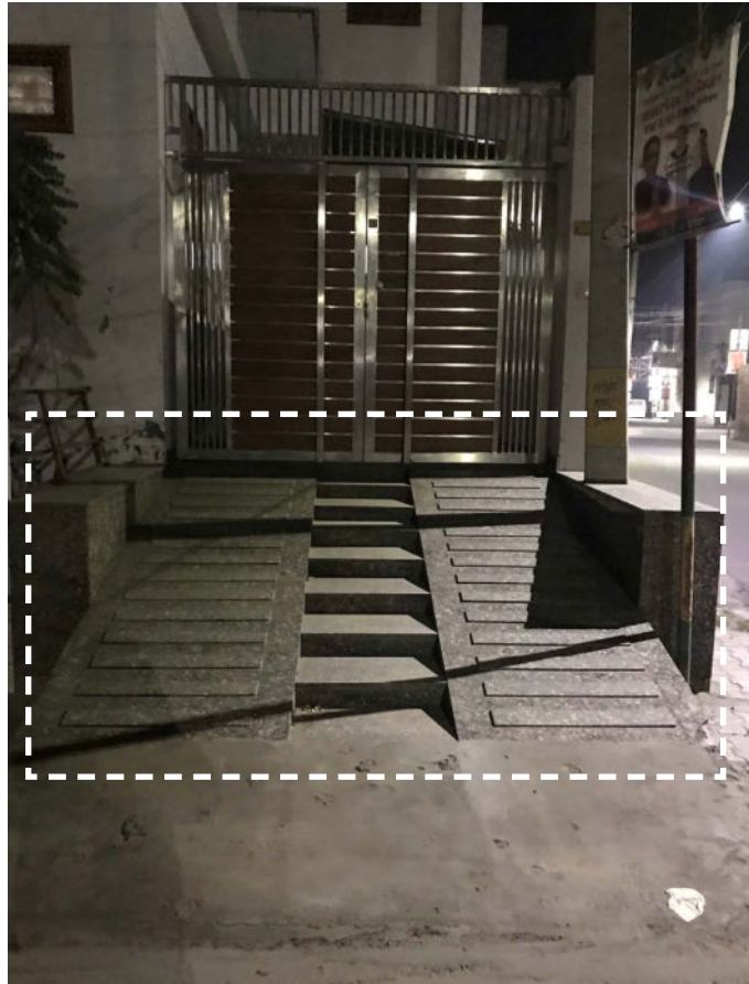
Image 2.14 Improper ramp detailing
