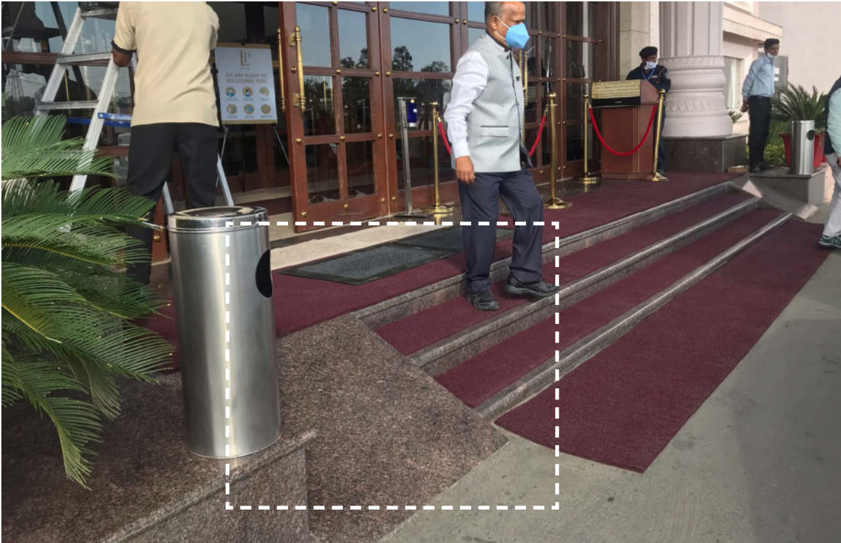
Image 2.7 Improper ramp gradient and slippery floor finish
