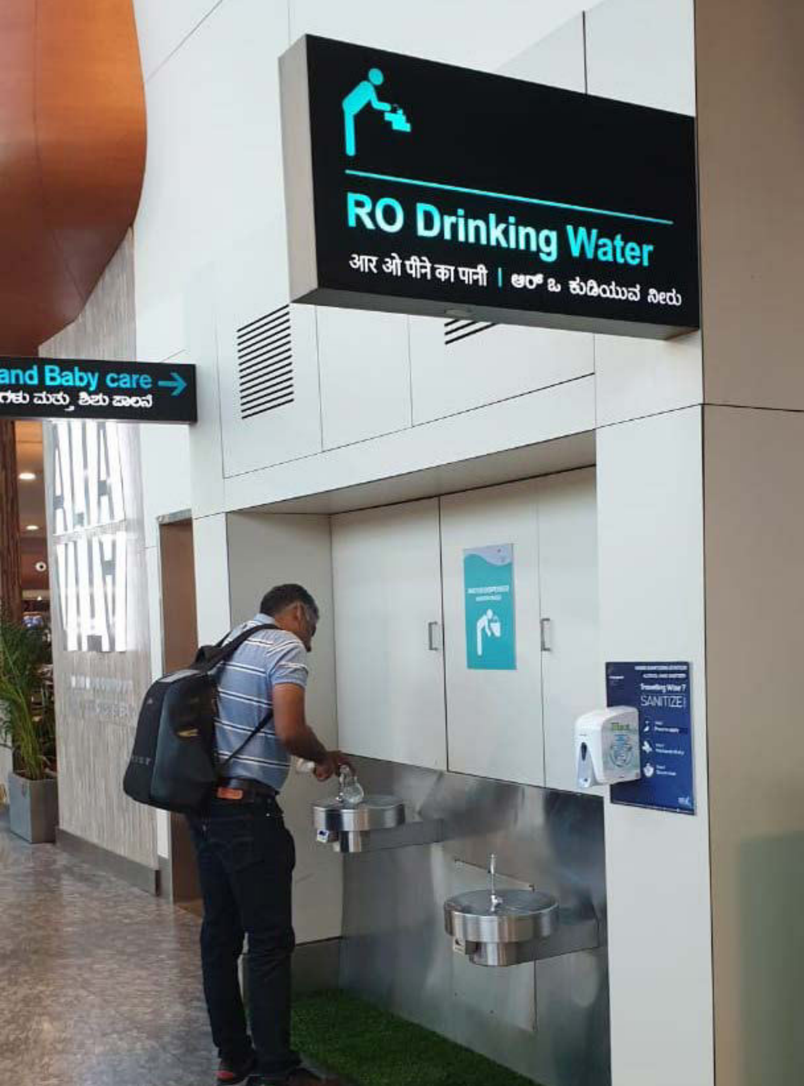
Image 4.13 Accessible Drinking water fountains Photo Credits: Shreya Shetty
