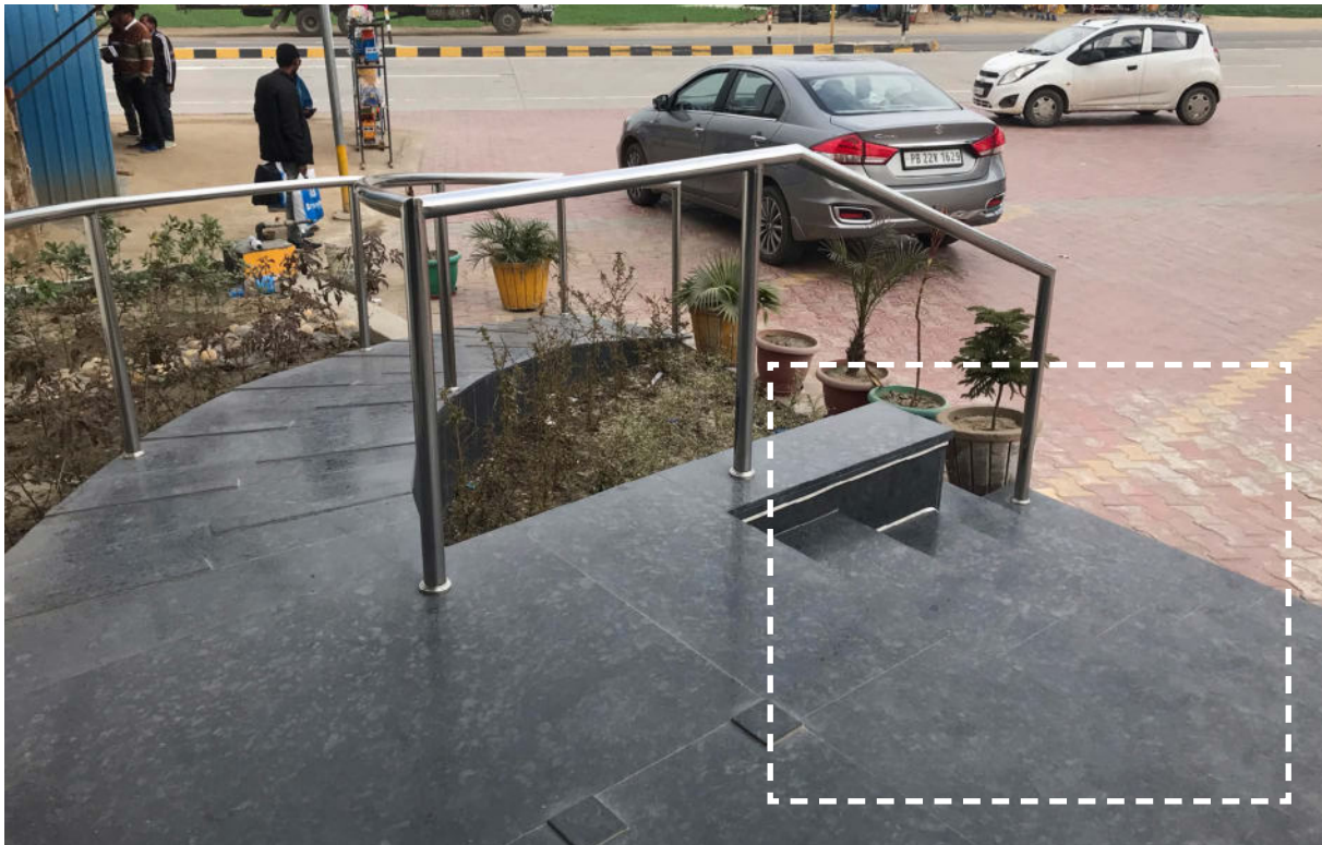
Image 2.10 Inadequate visual contrast
