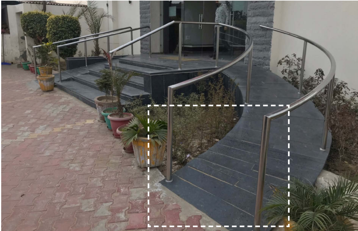
Image 2.9 Curved ramp with improper detailing and design
