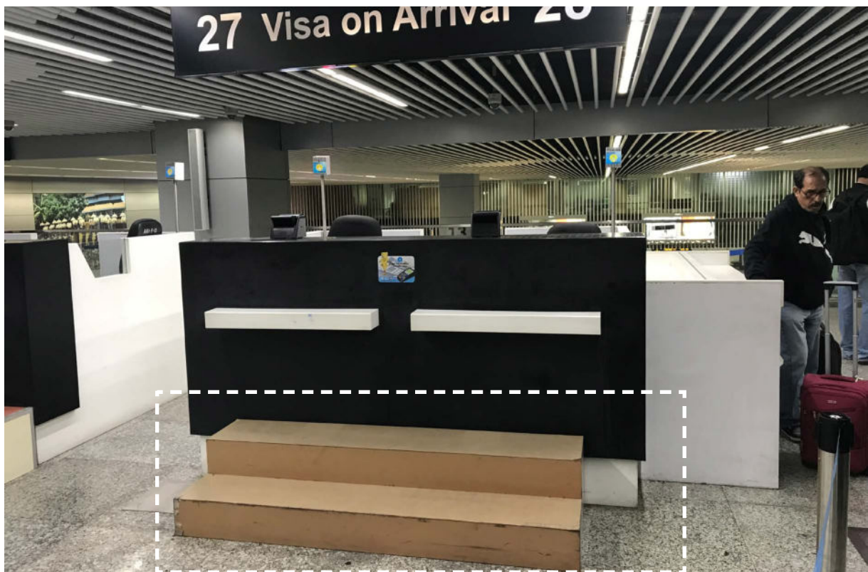
Image 2.25 Inaccessible counter heights
