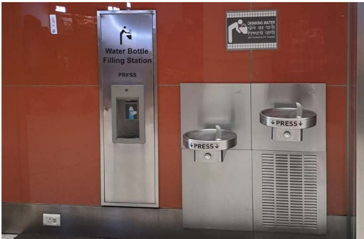
Image 4.12 Accessible Drinking water facility Photo Credits: Shreya Shetty
