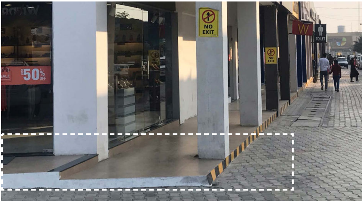
Image 2.15 Improper edge detailing of level change
