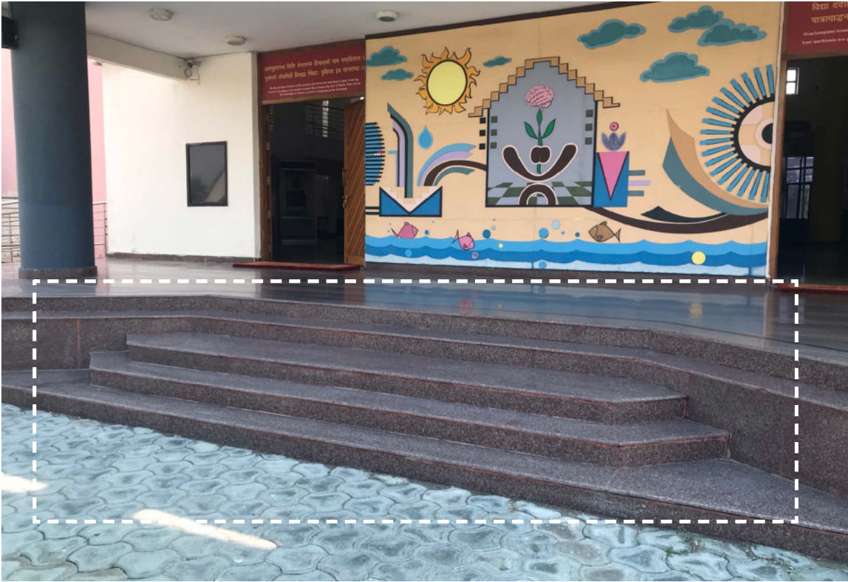
Image 2.3 Absence of adequate visual contrast in steps
