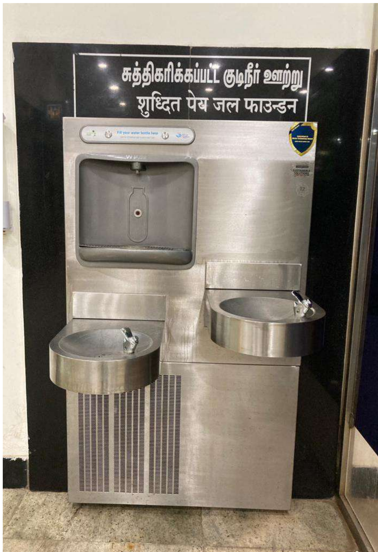
Image 16: Example of Drinking water facility with taps on two levels installed in Madurai Airport
