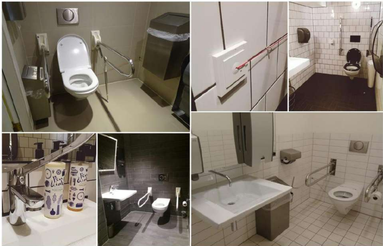
Image 13: Example of lever type tap, foldable grab bars, etc. in accessible toilet type A (Source: https://www.ableamsterdam.com/wp-content/uploads/2019/06/accessible-toilets-2-1024x662.jpg )
